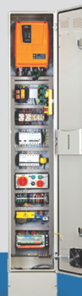
MRL Control Panel
